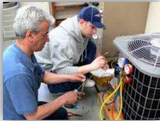
Air Conditioning /Heat Pump Professional
