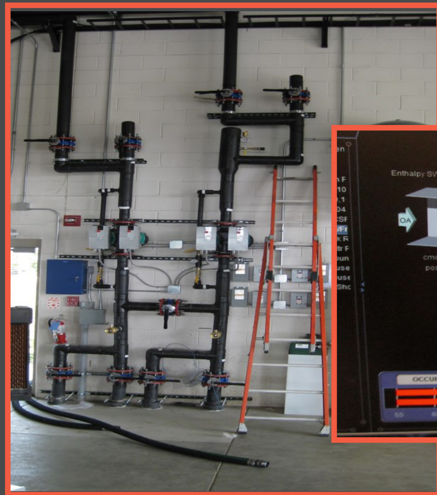
A supply return manifold.
